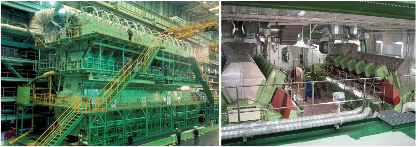
Fig. 2. a) World's largest diesel engine, RTA96-C . b) A ship's engine room .
